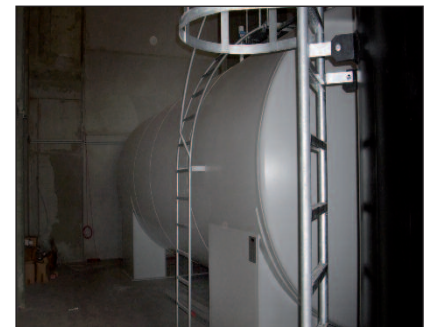
Harztank Resin tank
