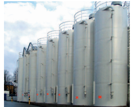
Rohstoff-Siloanlage Raw material silo plant
